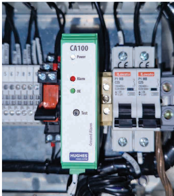
Installation in the motor drive cabinet
